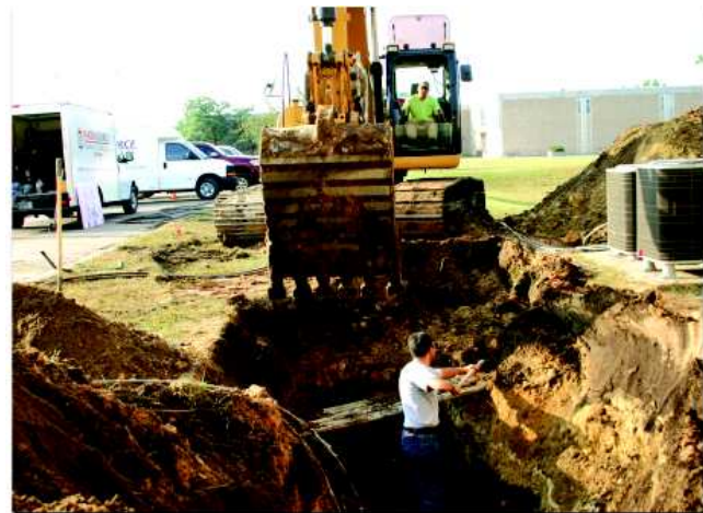
Three 170 ft. vertical loops are brought together in what is called a header shown here with Chad Green.
