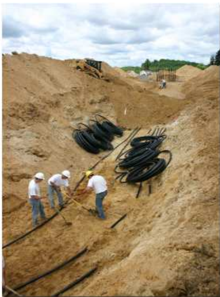
Water Source Heating and Cooling of Eau Claire installs the loop for Jackson Electric Cooperative’s new geo system. The inside work was done by Cargill, Inc. of LaCrosse.
